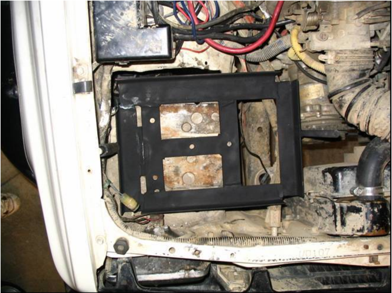
Figure 6. Near final installation of the “H” substructure and dual battery tray. Note the clearances with the A/C line, radiator, left headlight connector, left fender and fender well and the air tube. It fits though. Note ½” threaded rod at each of the tray for the battery hold down bar. The black material on the left threaded rod is rubber hose to protect the wiring harness right next to it. What’s not shown: four 5/16” carriage bolts to hold down the assembly (although the four holes are shown); the clearance into the left fender to clear the hold down bar and the closeout of the left fender well cutout, plus painting of the fender area.
